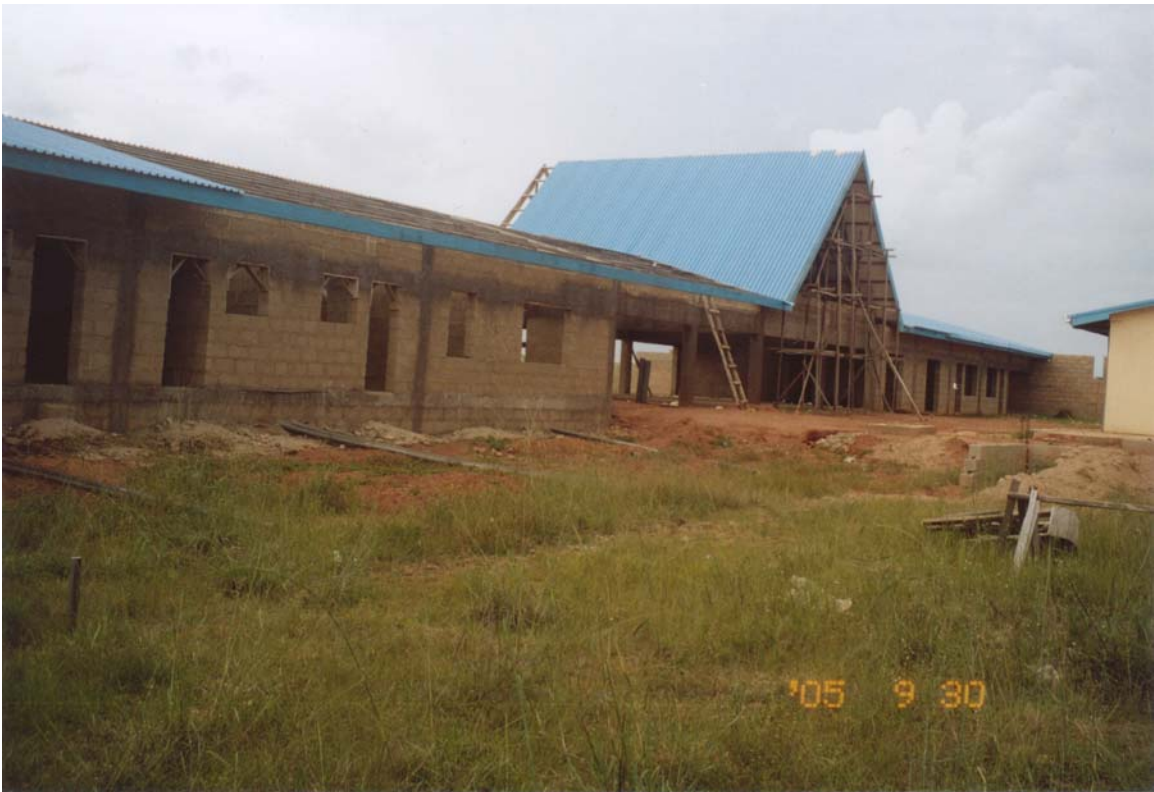
Foregrounds is construction of Hope Bible College classrooms. The Further end is being temporarily used as the literacy classrooms. Nigeria 2005, 2006.
